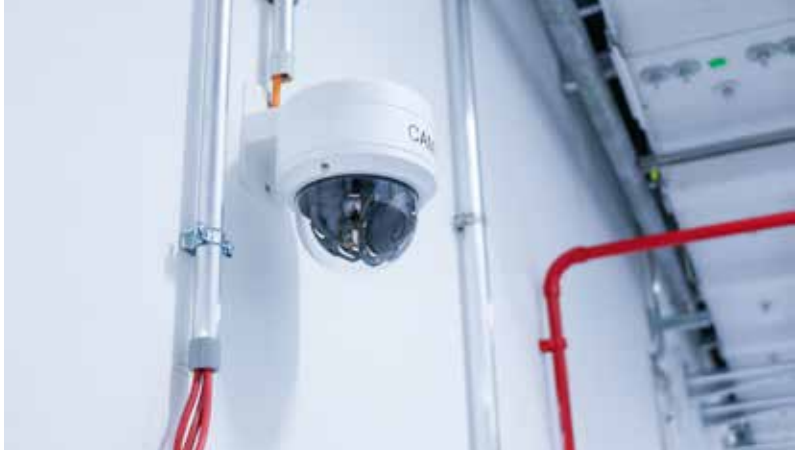
Comprehensive security and control system with video surveillance
