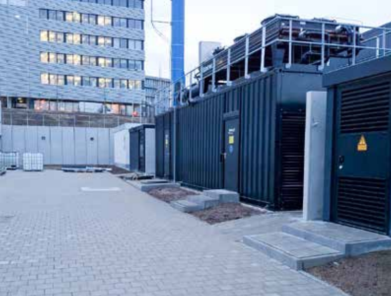
Technical containers with emergency power supply and cooling systems
