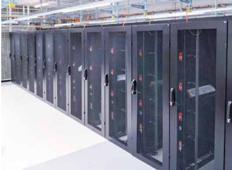
Server cabinets with 19" racks
