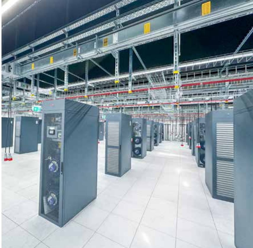
The IT components will soon move into the new data hall
