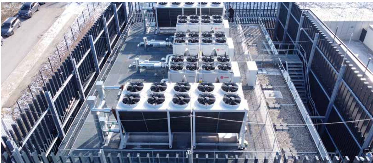
Chillers on the roof of the data center
