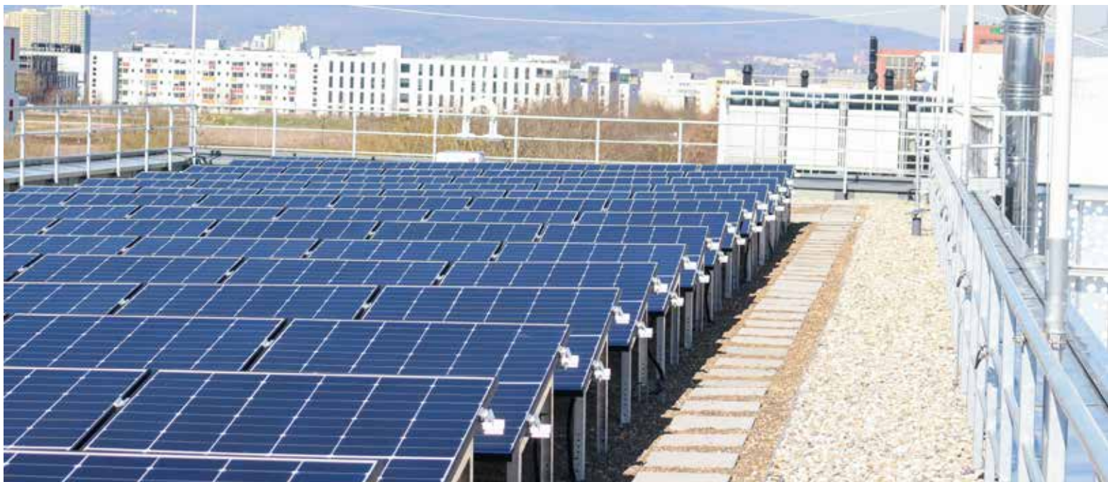
Photovoltaic panels on the roof for additional on-site power generation
