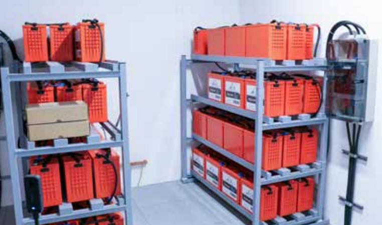
Battery storage room to bridge potential power failures
